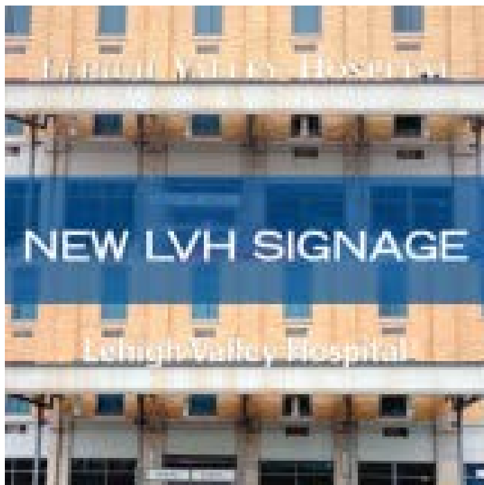
New Letters Brighten Entranceway at LVH-17th Street; Coming Soon to LVH-Cedar Crest
