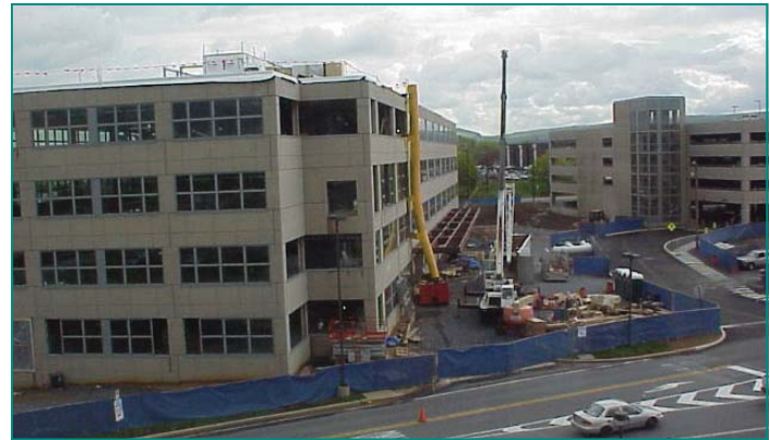
Work continues on the Center for Ambulatory Medicine. The majority of the building’s windows are now in place.
