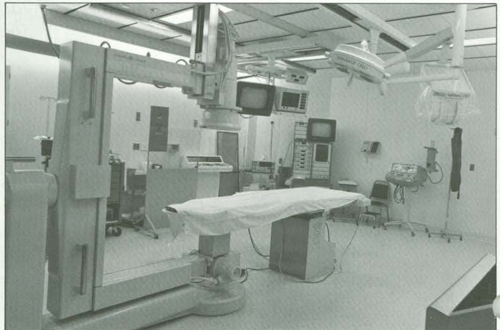
An overview of the new cardiac catheterization laboratory.
