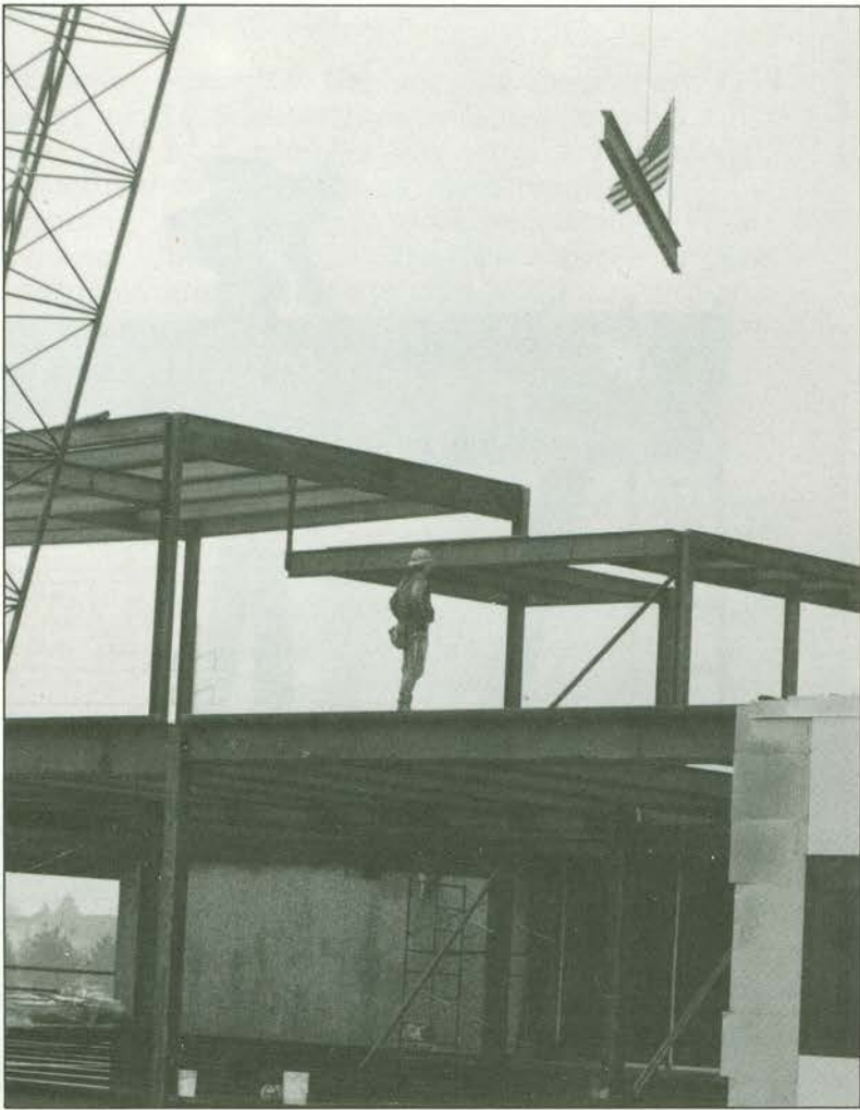
WEST WING FRAME COMPLETED: The final piece of framing steel for the west wing project was put in place on November 24. With the frame completed, the addition can be enclosed with prefabricated panels, and work will continue inside through-out the winter.
